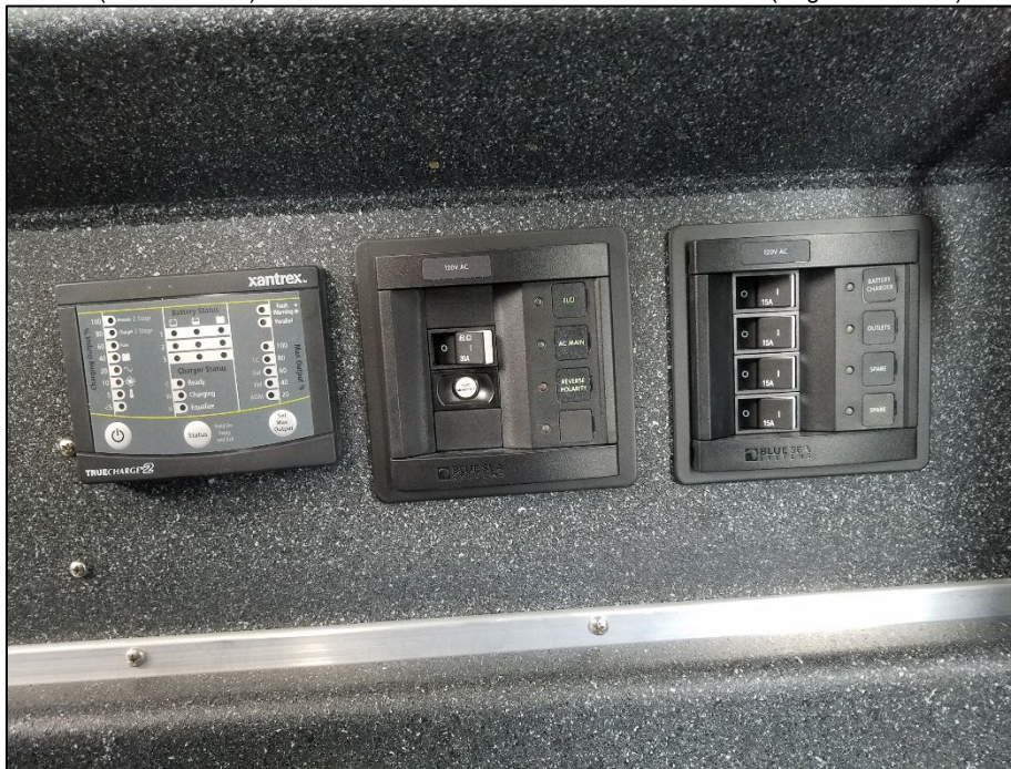
(Electrical switch panel)
