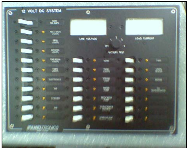
(Electrical breaker panel)
