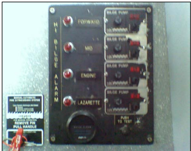
(Bilge pumps panel)
