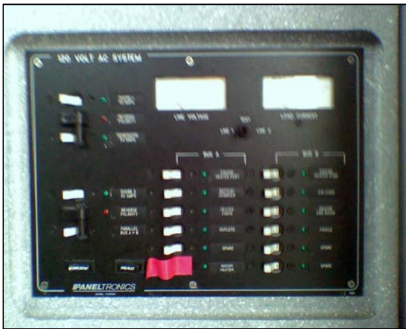
(Electrical switch panel)
