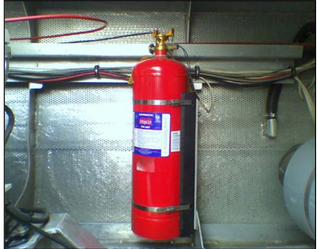
(Engine compartment fire suppression)
