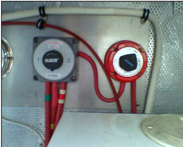
(Battery isolator switch engine compartment)
