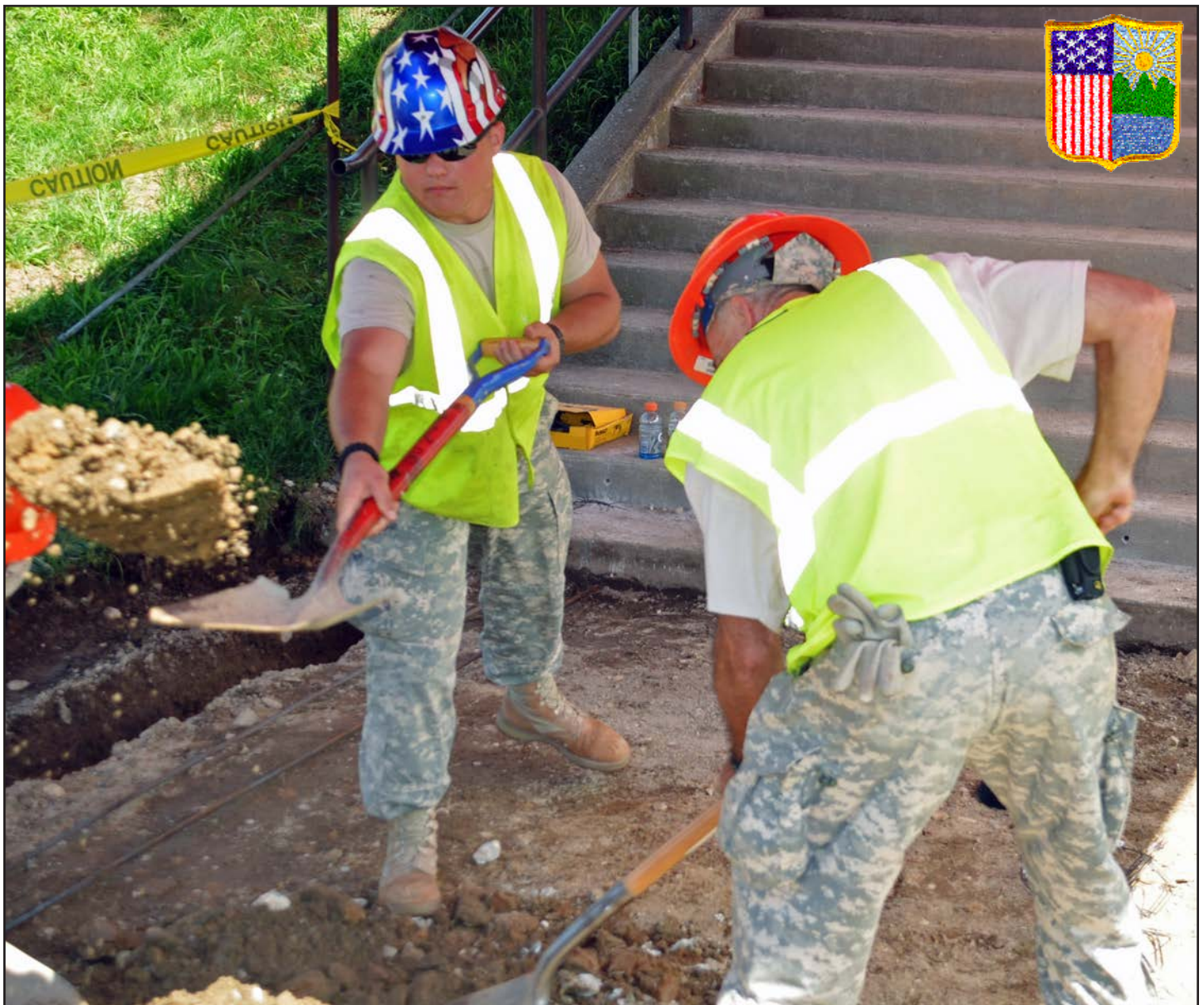
During their annual training in August, New York Guard troops level an area in front of Baker Hall so concrete can be poured. The work was one of the engineer projects New York Guard troops performed to improve Camp Smith. Photo by Capt. Mark Getman, New York Guard.
