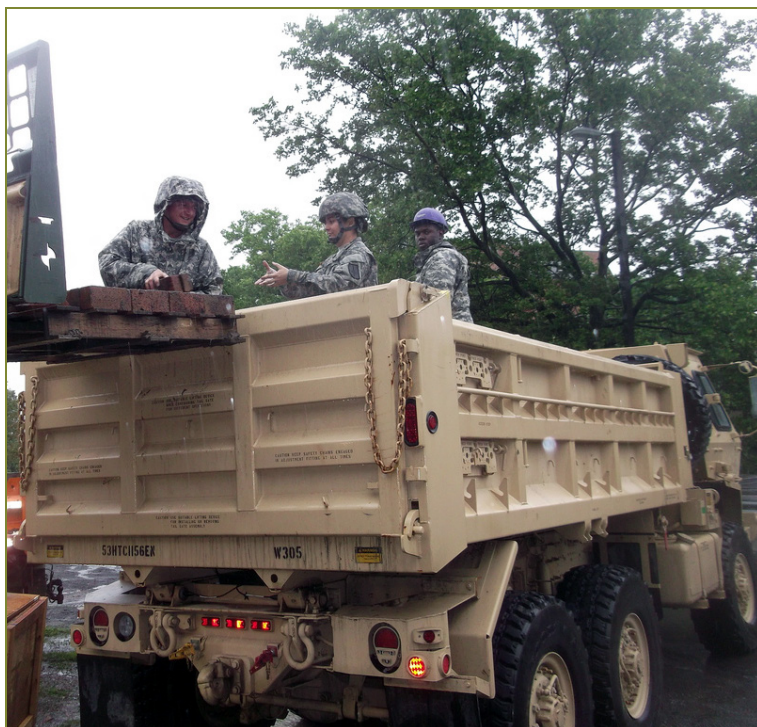
Soldiers of the 1156th Engineer Company load equipment as part of the final efforts in their community project June 13 to restore a former Erie Canal lock into a public park. The Soldiers provided a week-long effort during annual training each year since 2011 to remove debris from the abandoned lock, overgrown since 1911. Cohoes partnered with the Guard to remove the debris, install drainage and develop a walking path as part of the lock's conversion.
