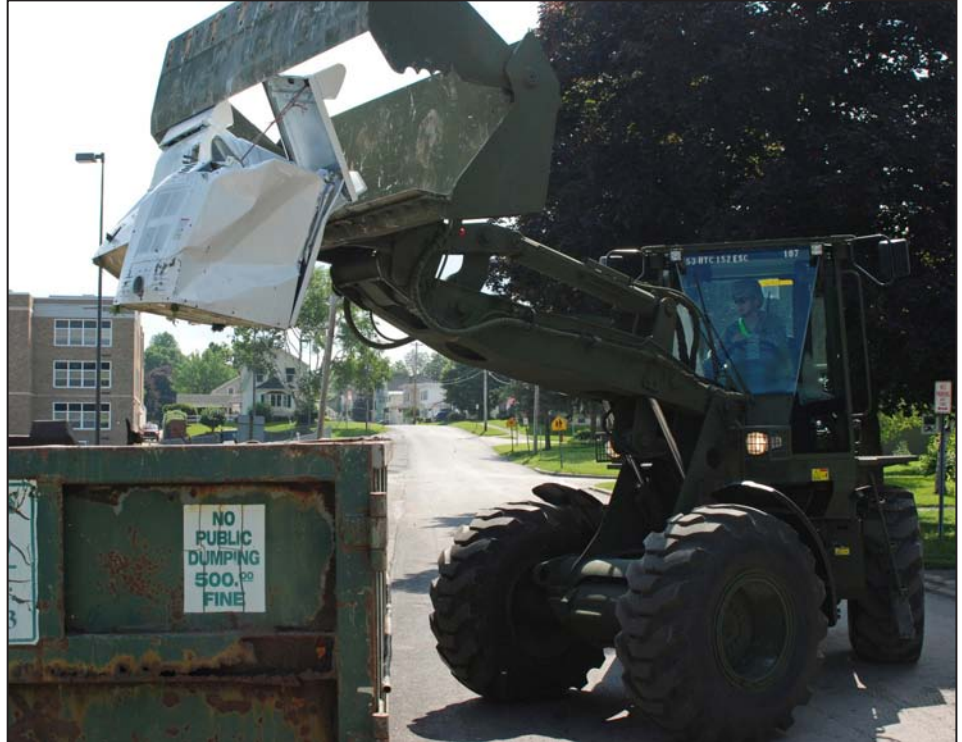
Sgt. John Johnson, from Stockton, N.Y., uses a front-end loader to drop flood-damaged appliances into a dumpster in Mohawk, N.Y. July 5. Johnson belongs to the Buffalo-based 152nd Engineer Company, one of the units called up to provide humanitarian assistance to flood victims and clear debris in towns like Fort Plain and German Flatts, N.Y. Soldiers helped dispose of flood debris from about 150 homes here by July 7. Photo by Sgt. 1st Class Raymond Drumsta, Joint Force Headquarters.
