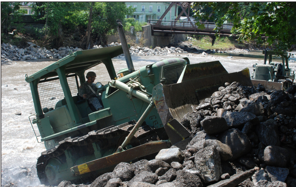
Pfc. Michael Bykowicz, from the Buffalo-based 152nd Engineer Company, uses a bulldozer to remove rocks and other flood debris from Otsquago Creek near Fort Plain, N.Y. July 4. In addition to other missions, the engineers removed an island of debris which had choked the creek’s flow. Bykowicz is from West Seneca, N.Y. Photo by Sgt. 1st Class Raymond Drumsta, Joint Force Headquarters.
