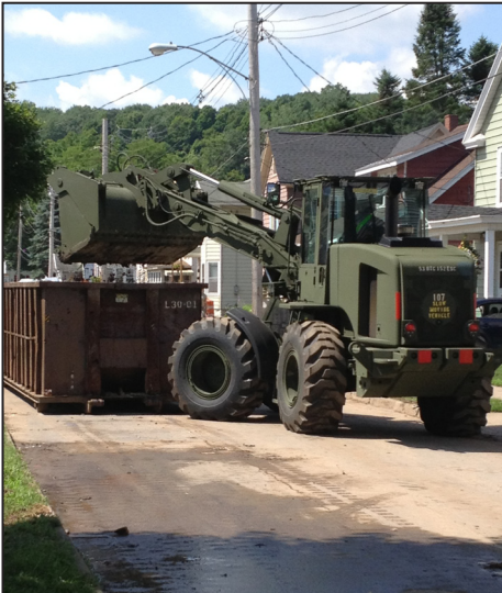
Engineers and Military Police Soldiers work together to help with debris clearance in Mohawk, N.Y. on July 3. Photo by Lt. Col. Christopher Panzer, Joint Force Headquarters.
