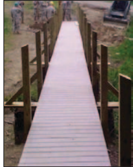
During their unit annual training this summer, Soldiers from the 1156th Engineer Company provided a construction platoon for the Boys and Girls Club of Schenectady to Camp Lovejoy in Altamont to construct a bridge, pavilion and some small "fix-it" projects around the camp. Photo by 1st Lt. Sean T. Gill, 1156 Engineer Company.
