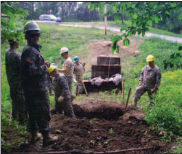
The early stages of construction of a footbridge over a drainage swale, using existing concrete footings left from the previous bridge. Photo by 1st Lt. Sean T. Gill, 1156 Engineer Company.
