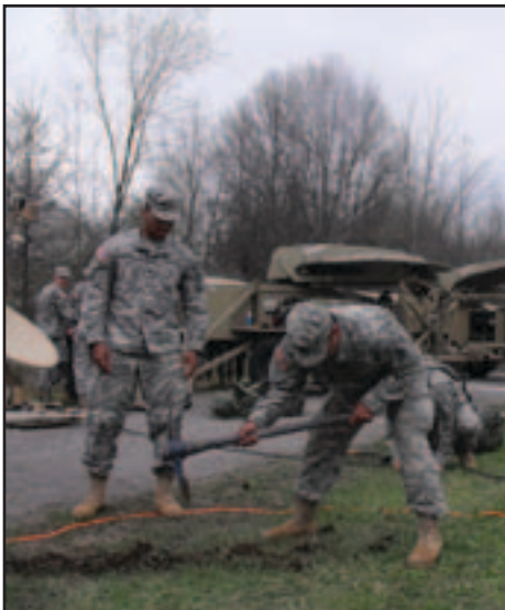
Soldiers with the 42nd ID Tac 1 dig a trench for the Hawkeye II cable reel.
