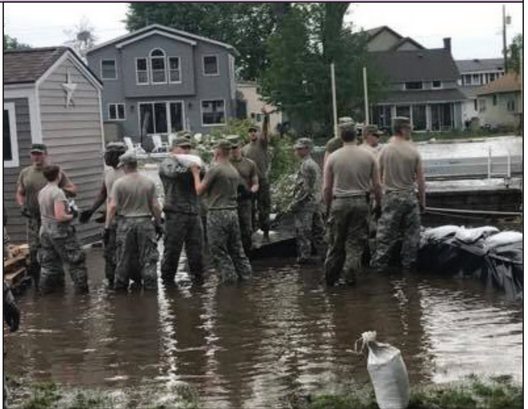
New York Army National Guard 105th Military Police Company Soldiers construct a sandbag barrier to protect property at Sodus Point, N.Y. from flooding due to rising waters on Lake Ontario on May 22. Photo by Sgt. 1st Class Patrick Belmont, 105th Military Police Company.
