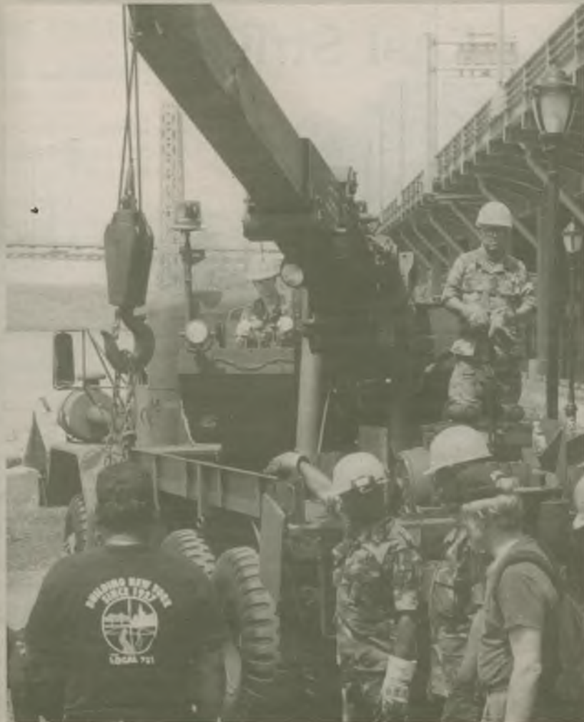
Private Rose Infanzon of the 145th Maintenance Company operates the crane on a 5-ton Wrecker during a recent GuardHELP project in Manhattan's Riverside Park to help lift heavy boulders onto a retaining wall along the Hudson River. The project began last Fall and resumed in May when Guard members rejoined local Union volunteers and NYC Park employees in restoring park facilities. The park is located on the West Side near the George Washington Bridge. Photo by Lt. Col. Paul Fanning
