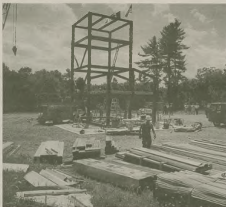
The steel frame of the fire tower goes up in the Columbia County town of Philmont. The tower will be used to train volunteer firefighters in Columbia County. Photo by Senior Chief Journalist Brian Bell.
