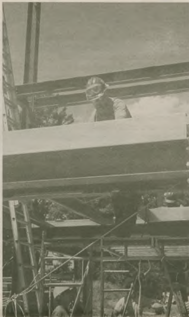
A seabee from the New York Naval Militia works on the steel frame fire tower. Photo by Senior Chief Journalist Brian Bell.
