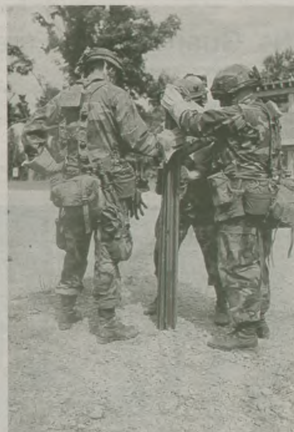
Members of the 427 Engineer Company emplace obstacles for an infantry check point. Photo by Spec. James Sylvester.
