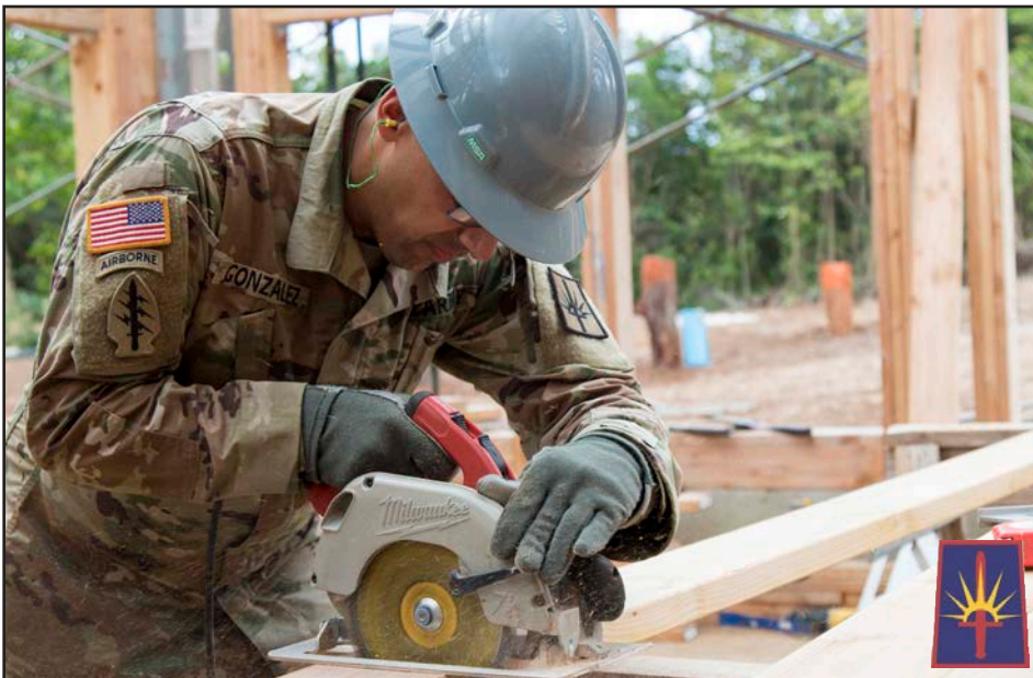
Sgt. Ronald Gonzalez, a wheeled vehicle mechanic assigned to the 1156th Engineer Company, 204th Engineer Battalion, uses a circular saw to cut a board that will be used for framing during Innovative Readiness Training at Girl Scout Camp Paumalu in Haleiwa, Hawaii, July 31, 2019.
