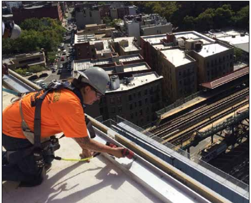
Tamara Gabbard working at 125th and Broadway in Manhattan, finishing 11th floor curtain wall covers. She is employed with Enclose contractors through the Local 580 Ironworkers Union as a first year apprentice.
