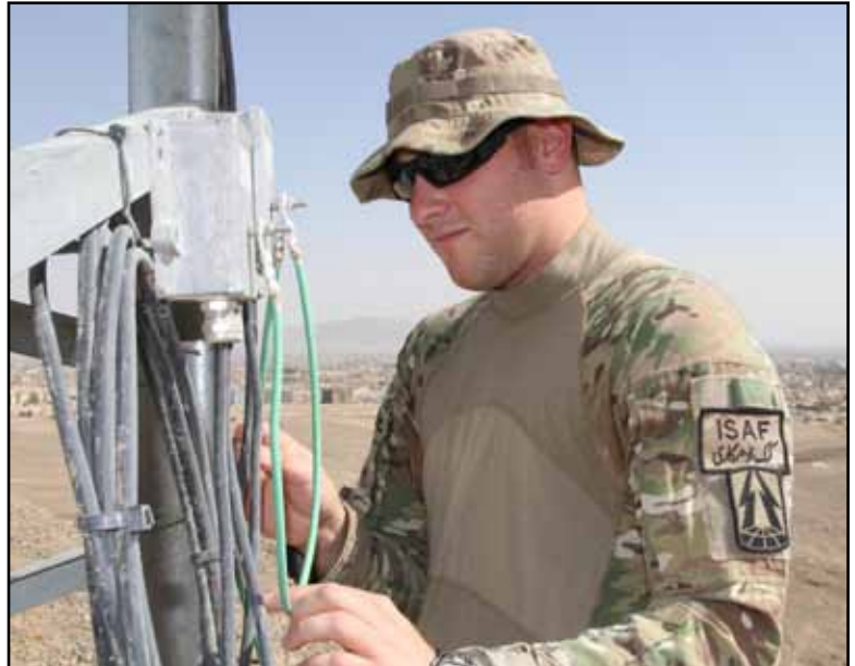
Senior Airman Matthew Perry, an engineer in the 213th Engineering Installation Squadron, 105th Airlift Wing, inspects wires at the base of a communications tower.
