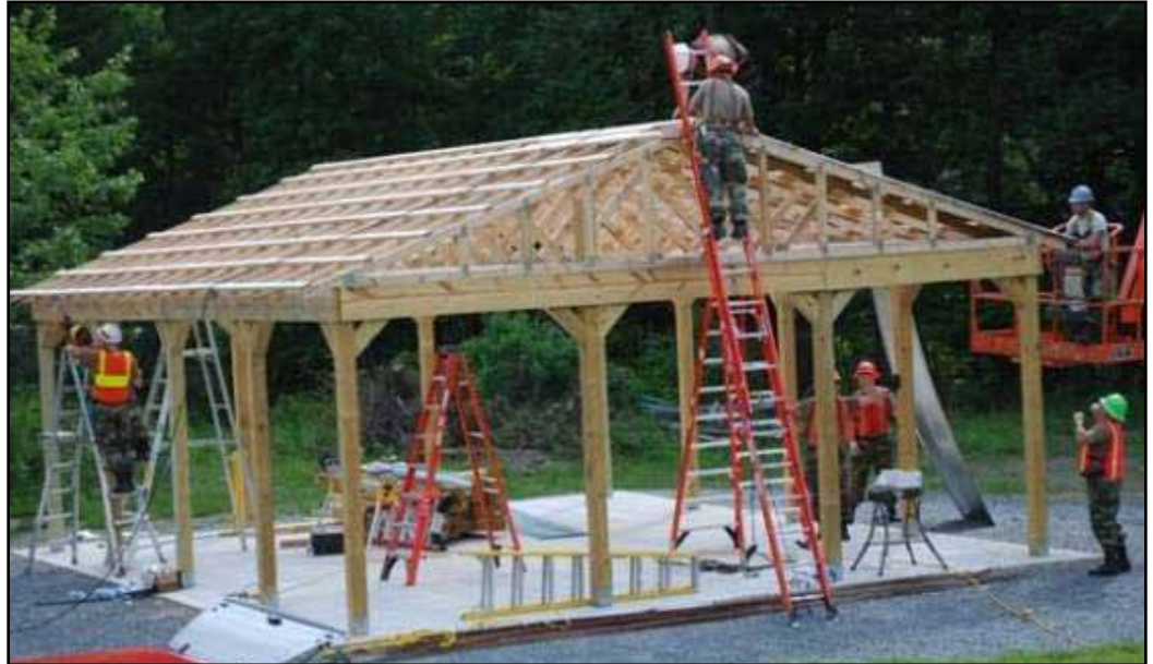
If you build it - they will train. Engineers of the New York Guard's 10th Brigade construct a roof over the Guilderland Training Area bleachers.
