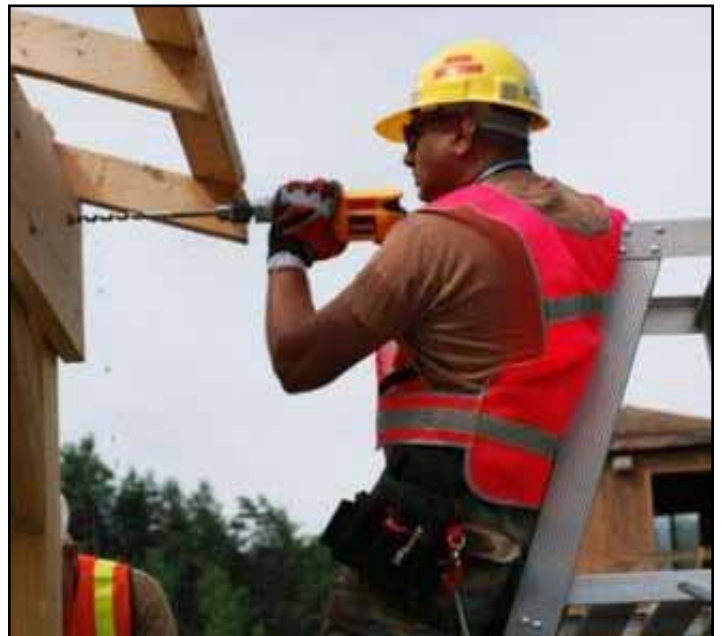
Command Sergeant Major Yatram Jagroop applies a power drill to the task of constructing the Guilderland range roof during the 102nd Engineer annual training at Guilderland Range near Albany, N.Y.
