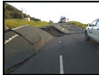
ABOVE: Buckling of a country-side highway near Christchurch, NZ. *
